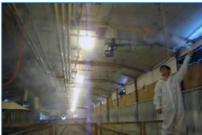
Figure 34: Using a smoke test to determine if airflow and operating pressure is correct.
