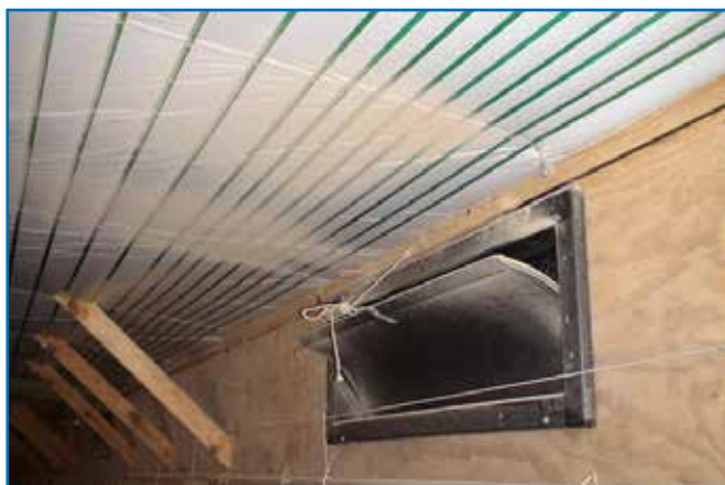
Figure 36: Example of a good quality air inlet.
