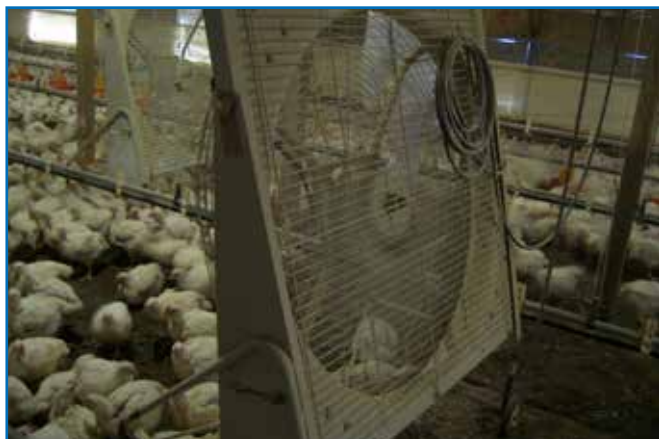
Figure 29: Circulation fans in a naturally ventilated house.
