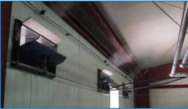
Figure 46: Example fogging system for a cross ventilated house.
